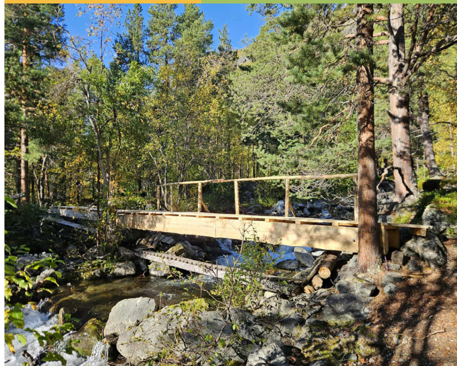
Building more resilient bridges because of water eroding the riverbanks. PHOTO: Asgeir Blixgård
